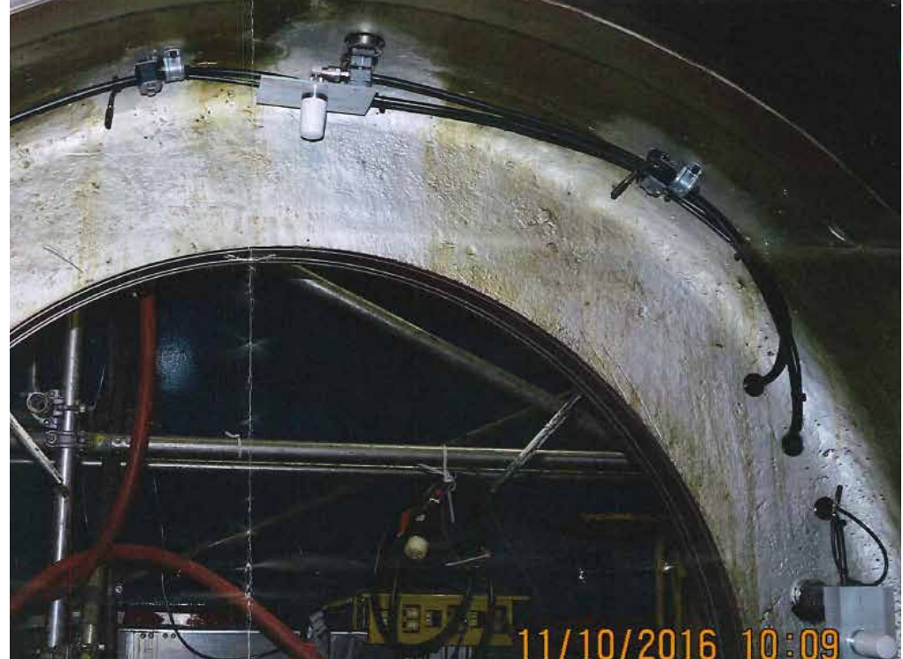
RF antenna systems attached inside bearing cover
